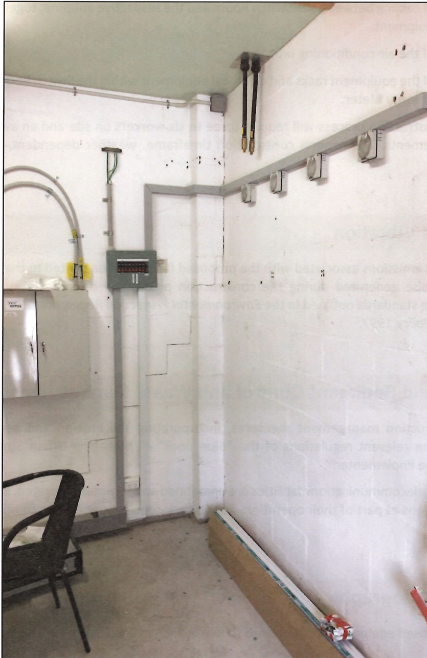
Figure 2: Proposed location of the equipment racks and electronic equipment within the existing Switch Room.
