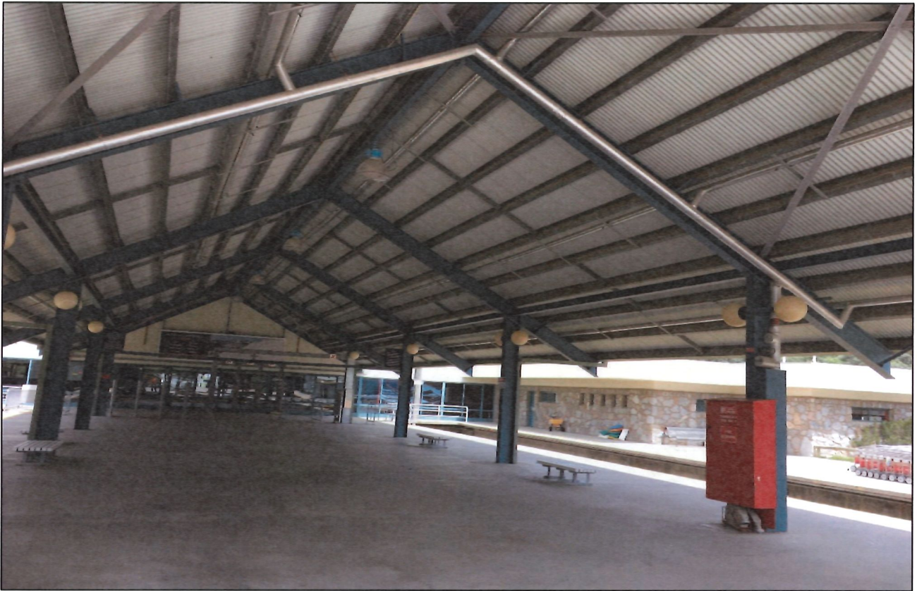
Figure 4: Proposed location of the Panel antennas at the western end of the major platform.
